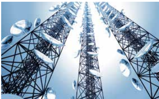
Telecommunications power supplies
